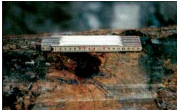
A leak in a ductile cast iron pipe developed over a number of years as the result of corrosion. Calculated annual water loss of 375,000 m 3 .
