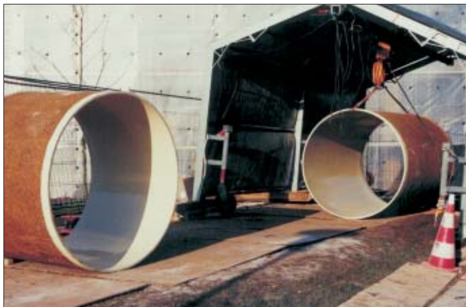
The pipes must be able to be installed via existing manholes and other constructions.
